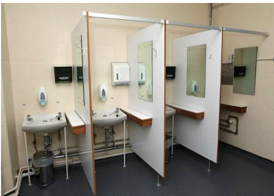
Non compliant toilet cubicles, Ailsa Hospital
