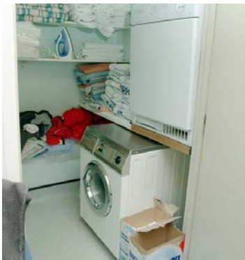
IPCU Laundry Room, Ailsa Hospital
